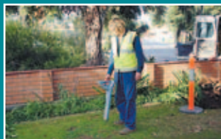
Pipe and cable locating and underground/floor leak detection services.
