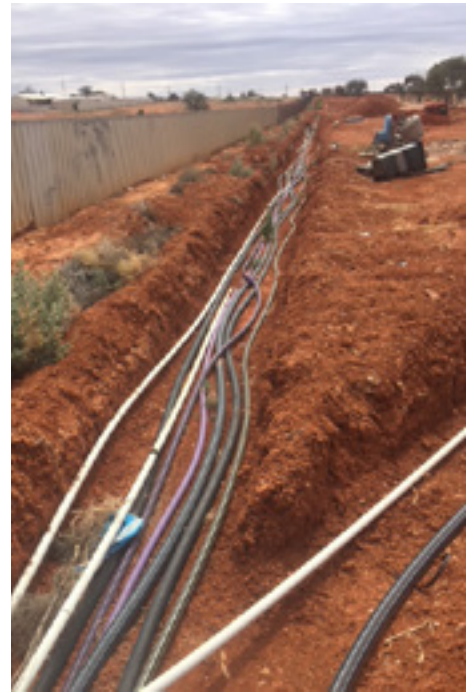
Underground services without correct separation.
