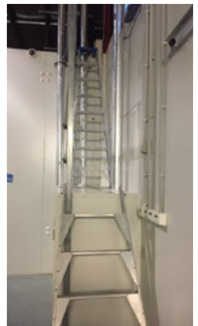
Equipment at height should have a permanent safe means of access (shown in 3 photos above)
