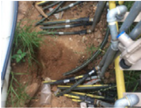
Examples of non-compliant installations (what a mess!)
